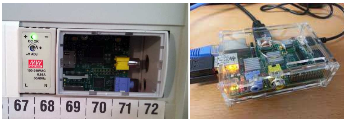
Figure 1: Left: The Raspberry PI mounted in a household’s electrical cabinet. Right: As a demonstrator. It is connected to the internet and offers interfaces for a wide range of sensors and actuators, including smart meters, wireless plugs and thermometers.
