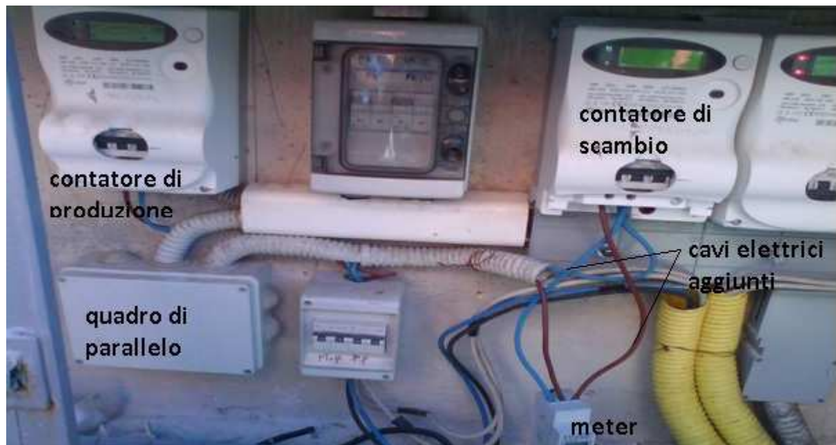
Figure 14: Image of the electrical cabinet of user CS-11 with an integrated SDM220-Standard type smart meter (compare with Figure 3, bottom left) for the measurement of PV energy flow depicted with meter.
