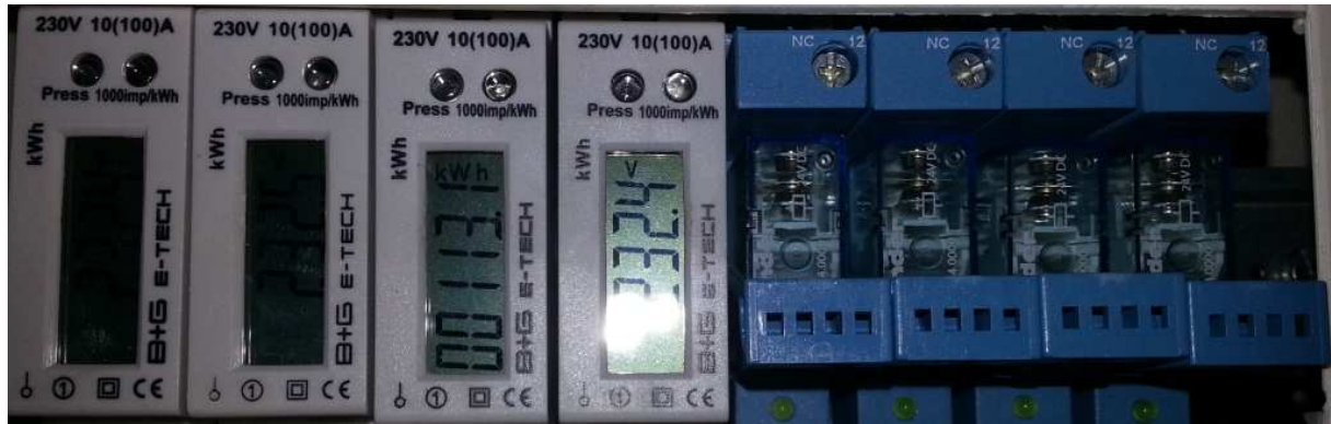
Figure 6: Array of four smart meters of type DRS110M (left) and remote controlled switches (right) in the electrical cabinet of user KN-10.
