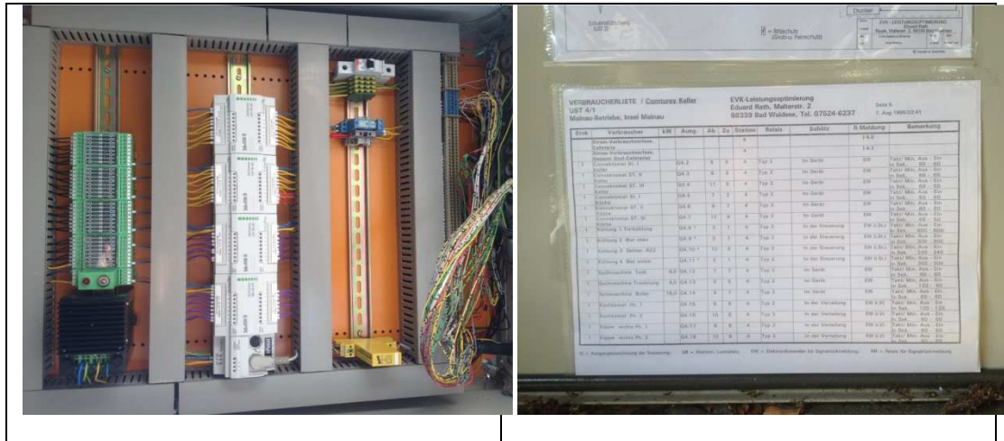
Figure 13: Installation inside the electrical cabinet.
